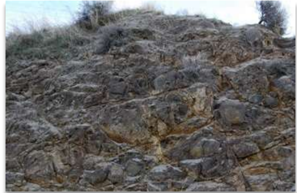
Figure 4. Outcrop of Ice Harbor basalt along the City View portion of Yakima Bluffs.
